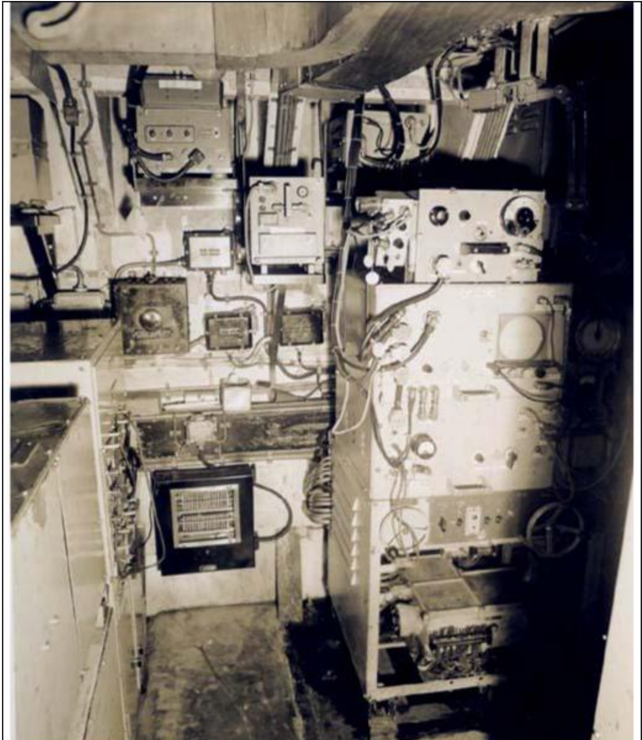
293M Office. After bulkhead: 293 transmitter; modulator; On the port bulkhead, 253P IFF (extreme left of photograph) 242 IFF responder, performance meter, modulator and mixer; Receiver panel L26, with wavemeter G82A and anti-wave clutter unit; AQR aerial control table (front cover removed to show control unit 20-H). (RCN photo # HS1749-54)
